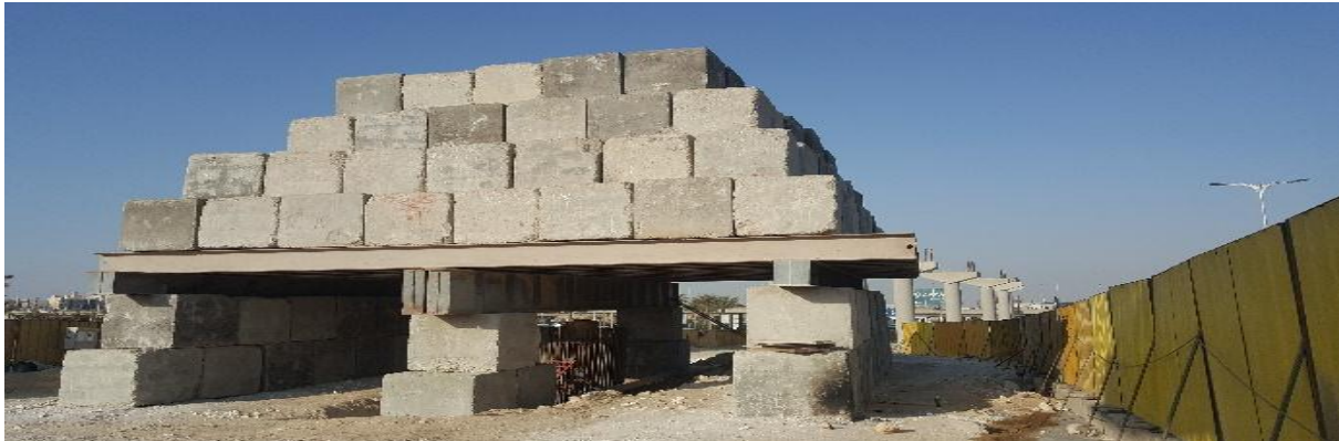
Fig. 4 Field photo of axial static load test, (The Arab Contractors, Foundation department, 2020)
